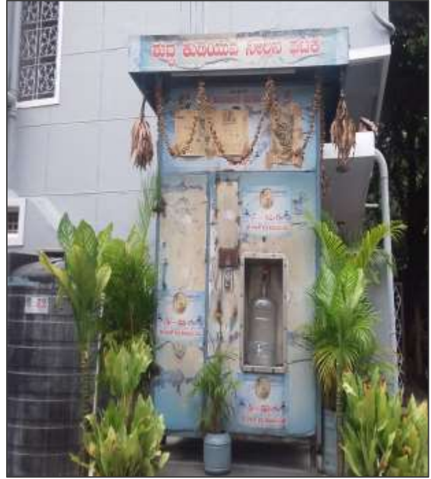
2. Clean Drinking Water Unit at Goripaliya Minority Colony of BBMP Warda No-137
