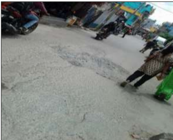
1. Uneven roadwork in BBMP South
