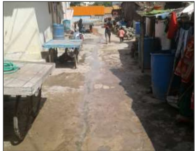
2. Proper space for drainage alongside the road was not provided in Lingasugur
