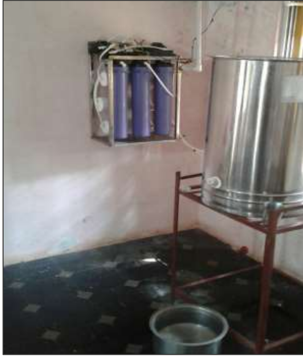
1. Water filter installed in Bellary not in use
